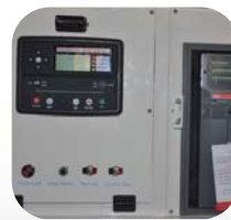
Control Panel & MCB
